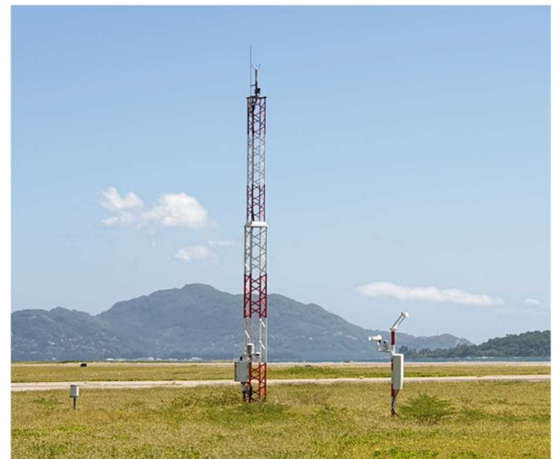
Figure 4: New technology weather measuring and monitoring equipment at Mahé International Airport Seychelles (2019)
